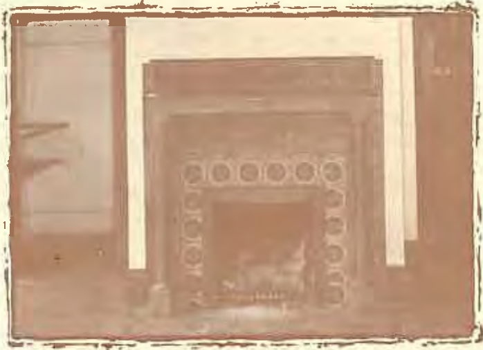
Character defining features such as historic fireplaces should be retained and preserved.
