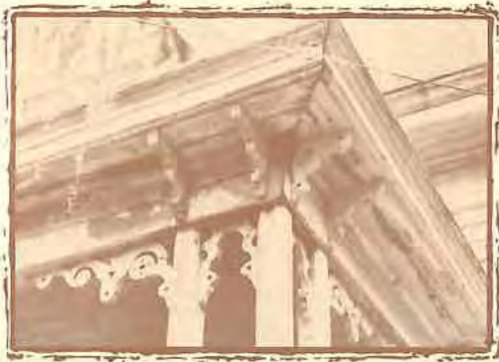
Some problems are very obvious, such as this rotting porch trim.
