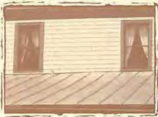
APPROPRIATE Standing seam metal is a common roofing material in Tallahassee, and should be replaced in kind when necessary.
