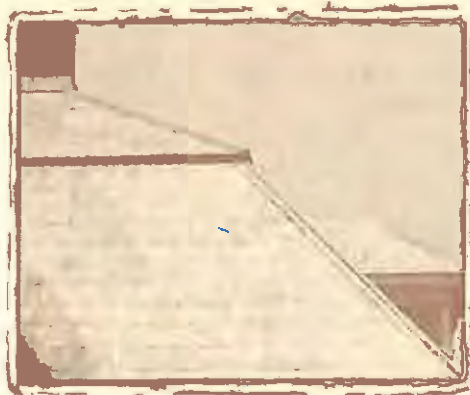
APPROPRIATE This pressed metal shingle roof is an important feature of the building.
